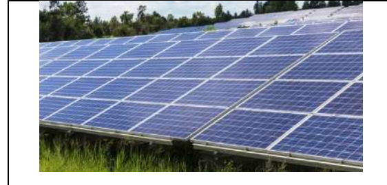
Fig.5 Polycrystalline Solar Panel [17]
